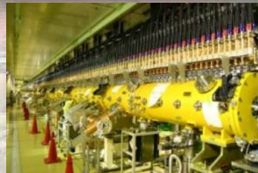
DTLs in the linac tunnel
