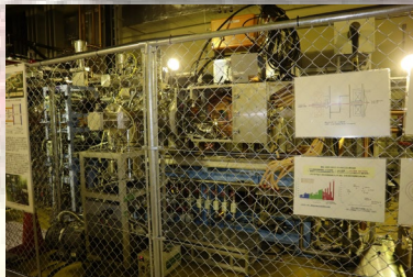
H - ion source in the linac tunnel
